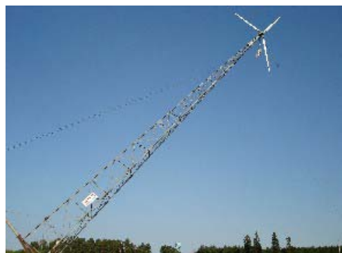
This picture shows the tip-up of the 120-foot Jacobs wind turbine tower.
