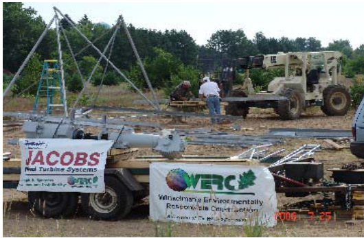
The tower assembly has just begun. In the foreground on the trailer is the turbine/generator waiting to be put into place when the tower is nearly complete.
