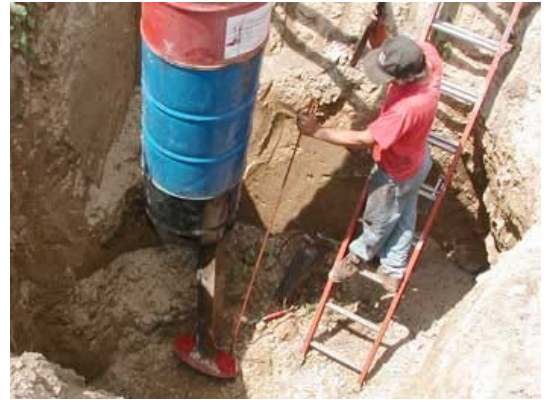
Pier foundation view Rebar will be welded in steel form for added strength.
